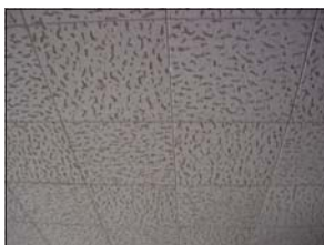
Floor and ceiling tile installed prior to 1980 is presumed to contain asbestos.
